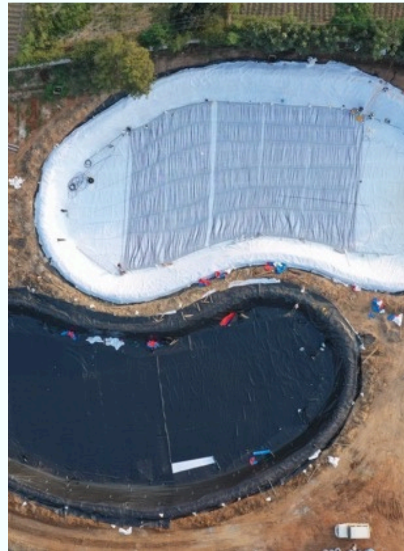
Aerated Wetlands for sewage treatment
